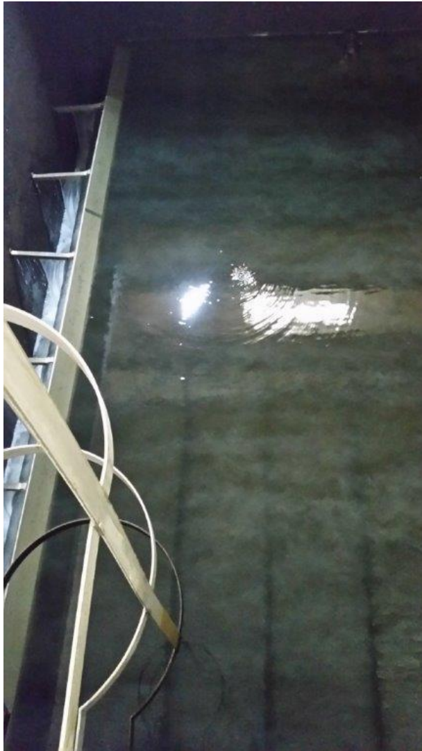
Photograph No. 1: Bubbles in the filter (seen across each filter.)
