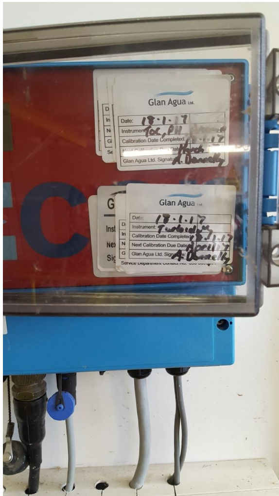
Photograph No. 2: Turbidity monitor no. 3, out of date calibration sticker.
