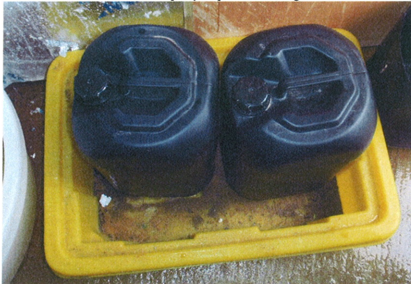
Photograph 2 – Bund holding two 20 L drums of Sodium Hypochlorite. Bund adequacy requires checking.
