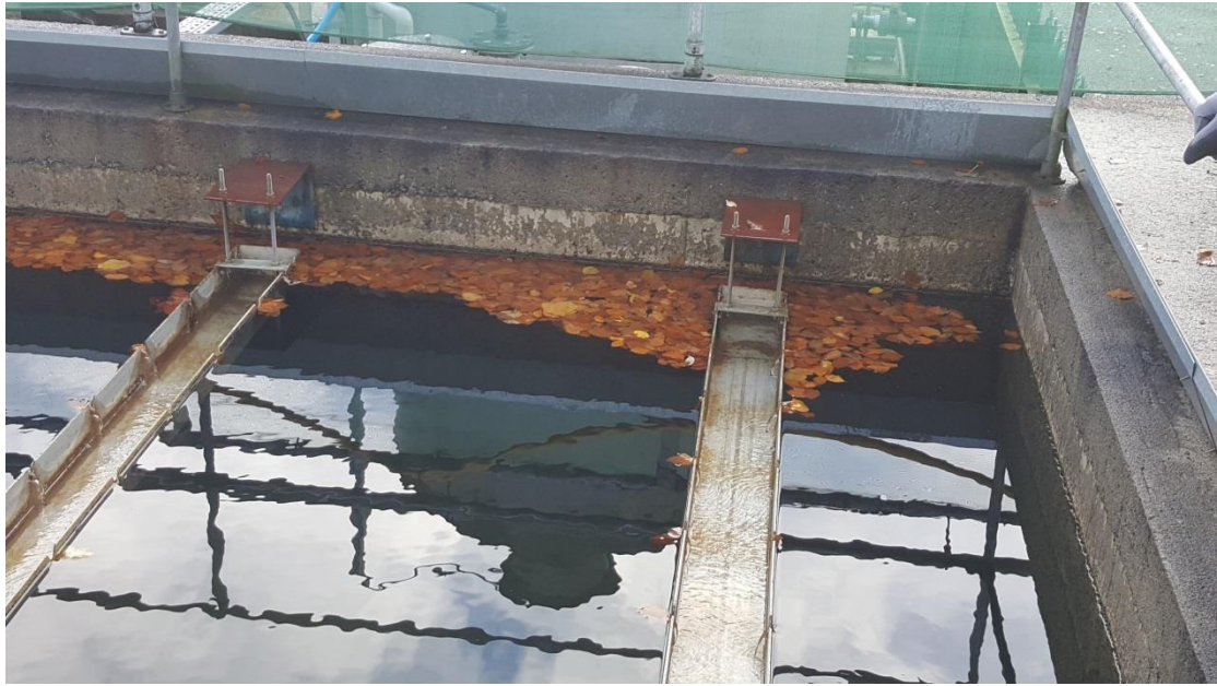
Photograph No. 1: Leaves on surface of Clarifier
