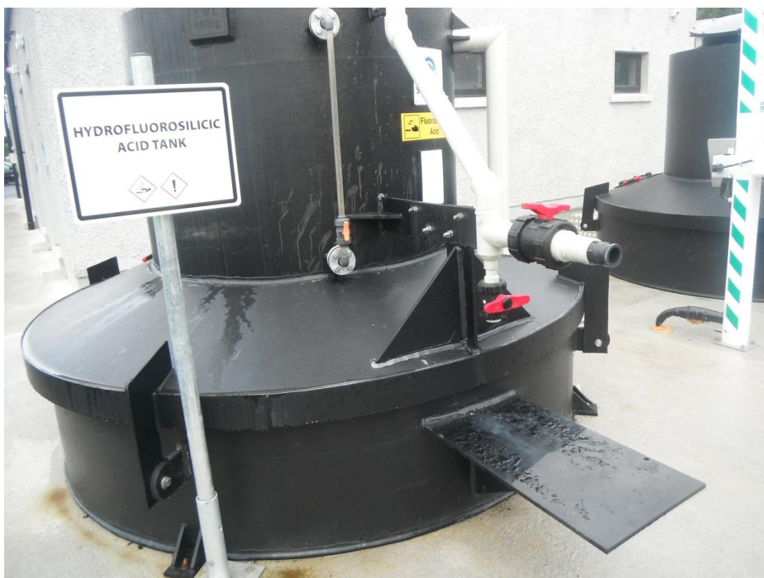
Photograph 1: Example of delivery pipe to bulk storage tank not within bunded area.
