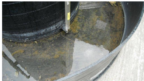
Photograph 2: Water in PAC bund.
