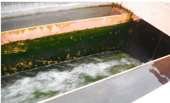
Photograph 1: Algae on filter channel and walls.
