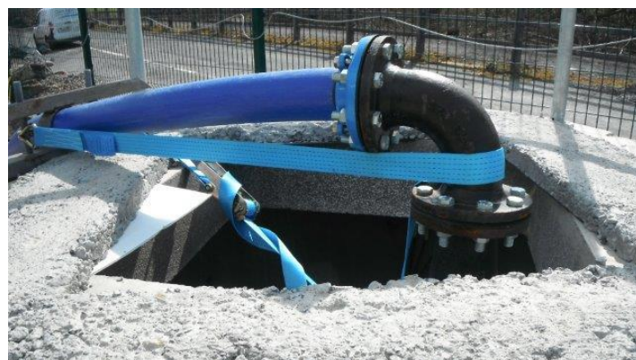
Photograph 3: Operational borehole without locked access hatch.
