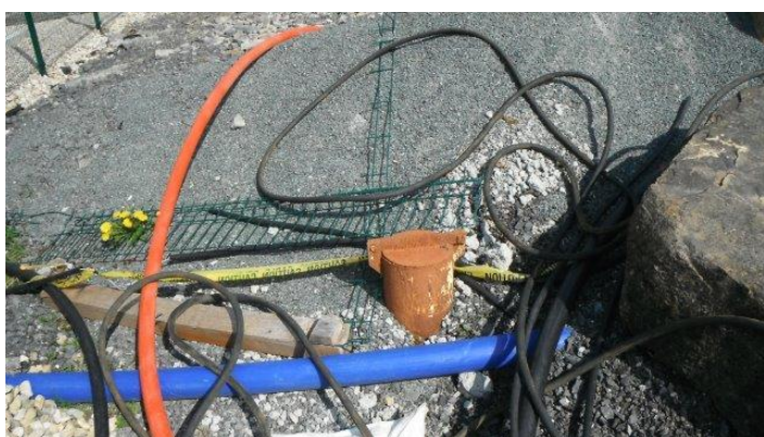
Photograph 2: Borehole that served the Hughtestown supply prior to October/November 2014 with gravel and other materials surrounding the unsealed well.
