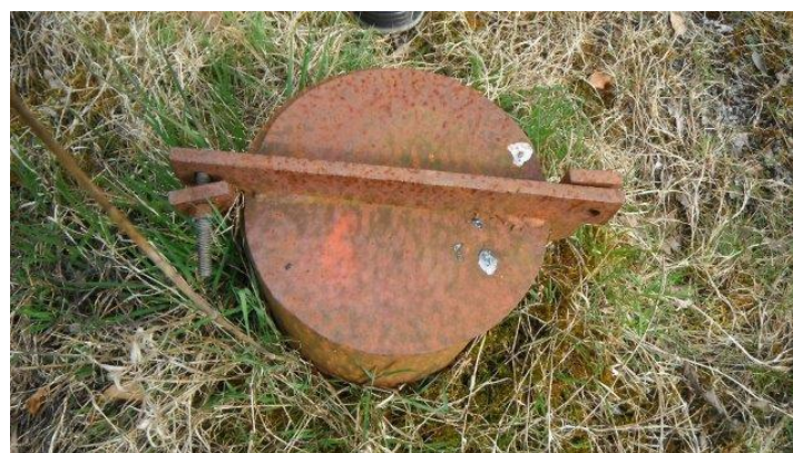
Photograph 4: An old trial well that should be decommissioned.
