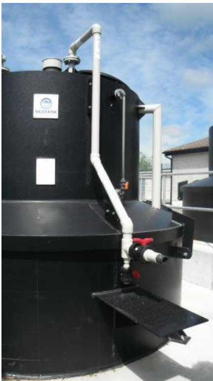
Photograph 2: Example of delivery pipe to bulk storage tank not within bunded area.
