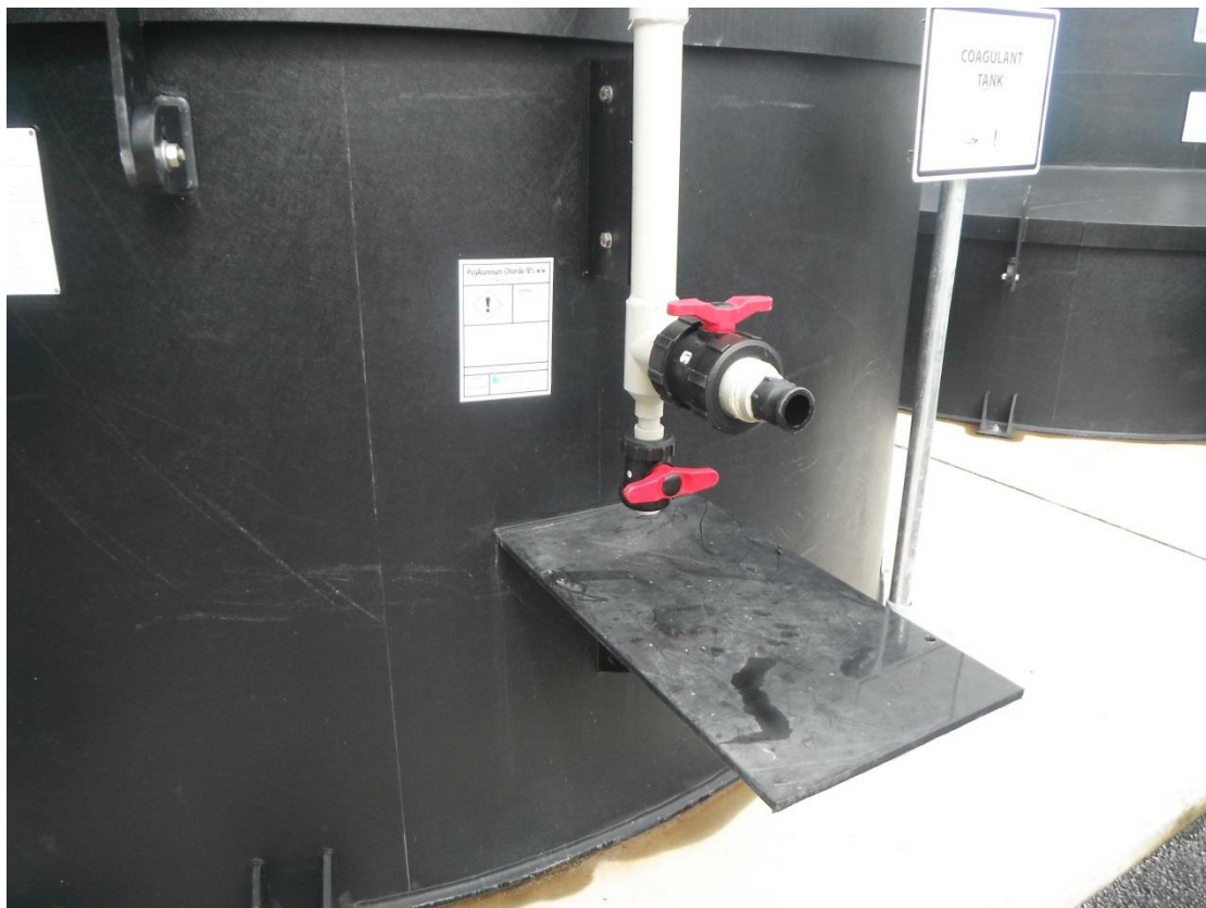
Photograph 1: Example of delivery pipe to bulk storage tank not within bunded area.
