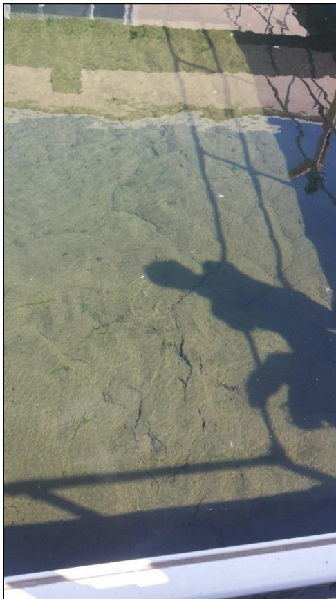
Photo 4: Cracks in filter media (Filter No. 5)
