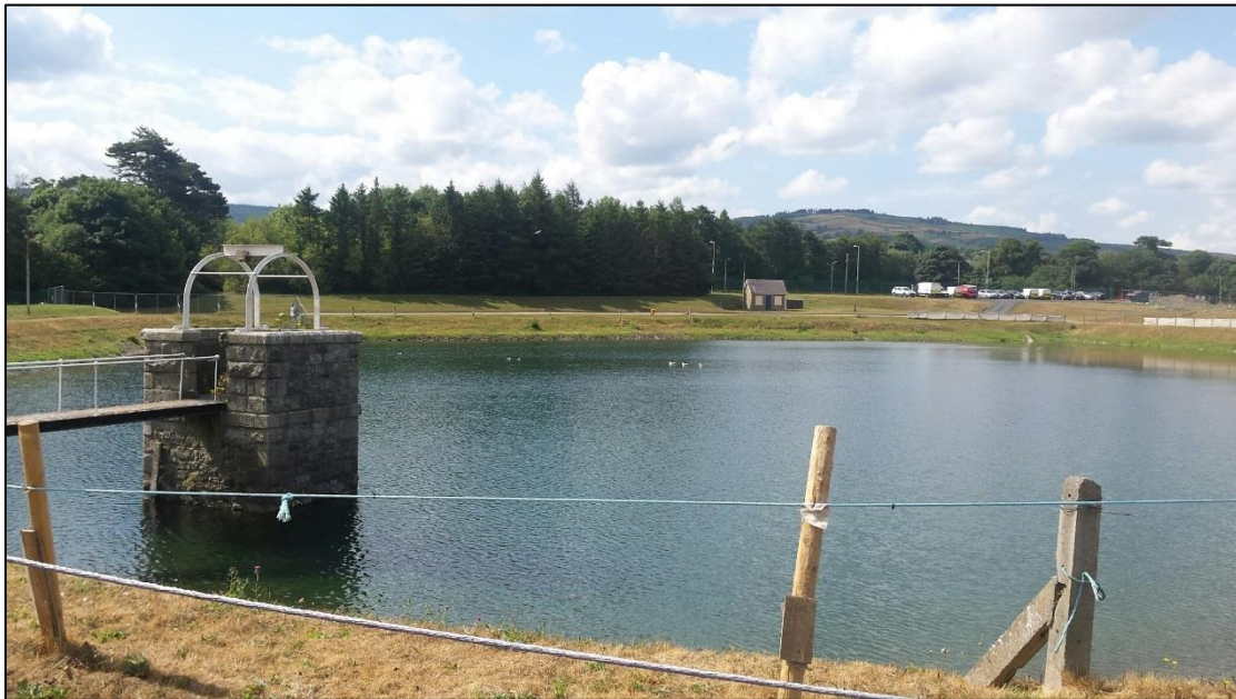
Photo 2: Open storage of treated water still in use on the day of the audit (note birds present on water surface)
