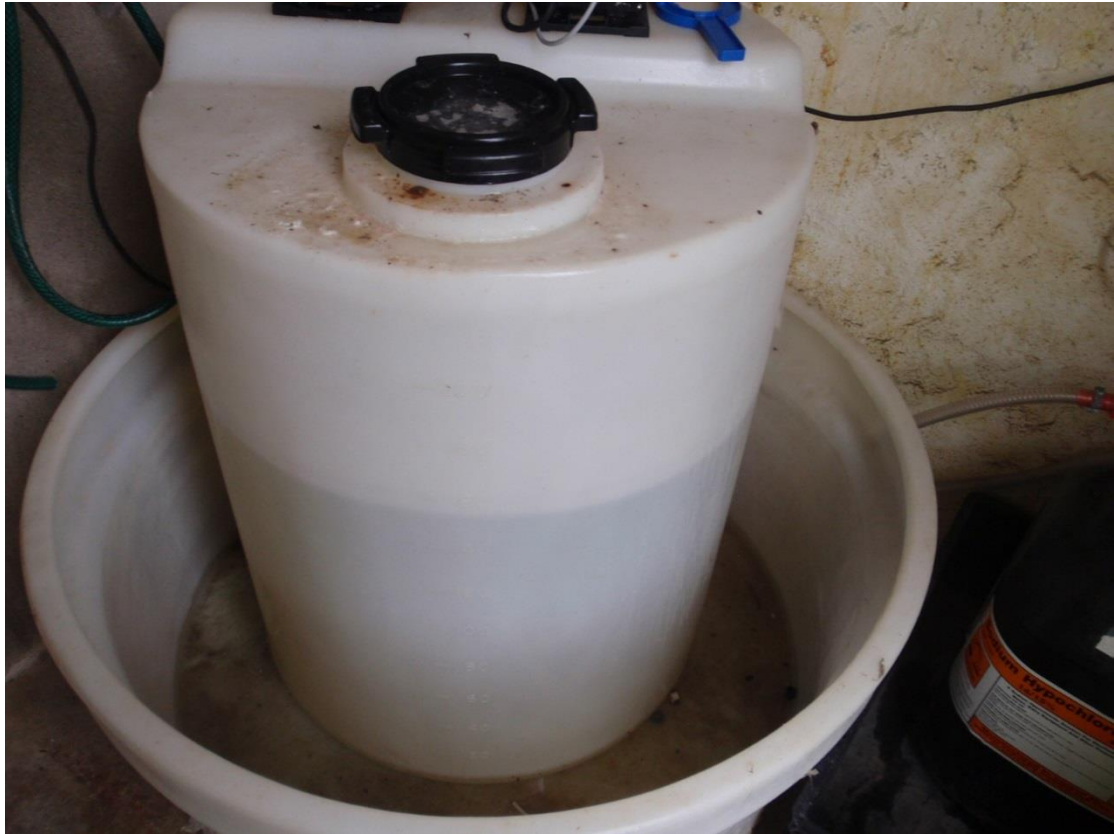
Photograph No.1 : Build Up of Liquid in Chlorine Day Tank Bund.
