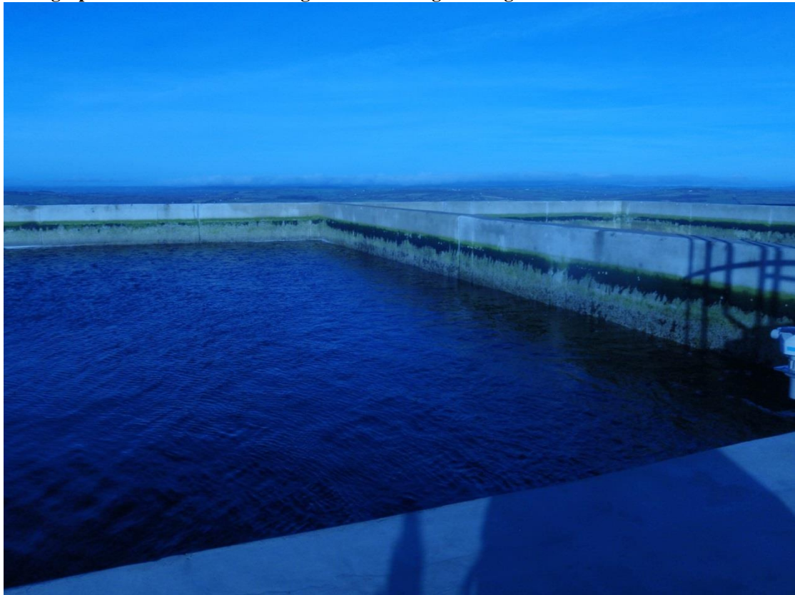
Photograph No. 1: Raw Water Storage Tank Showing Staining on Walls
