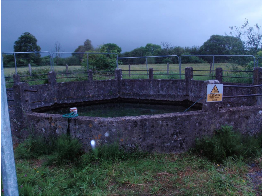
Photo No. 1 – Security Fencing Issue At Spring Chamber
