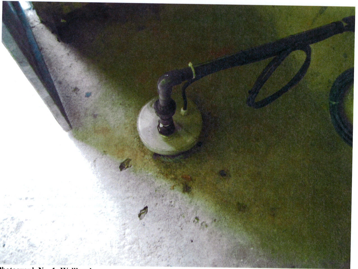
Photograph No. 1: Wellhead
