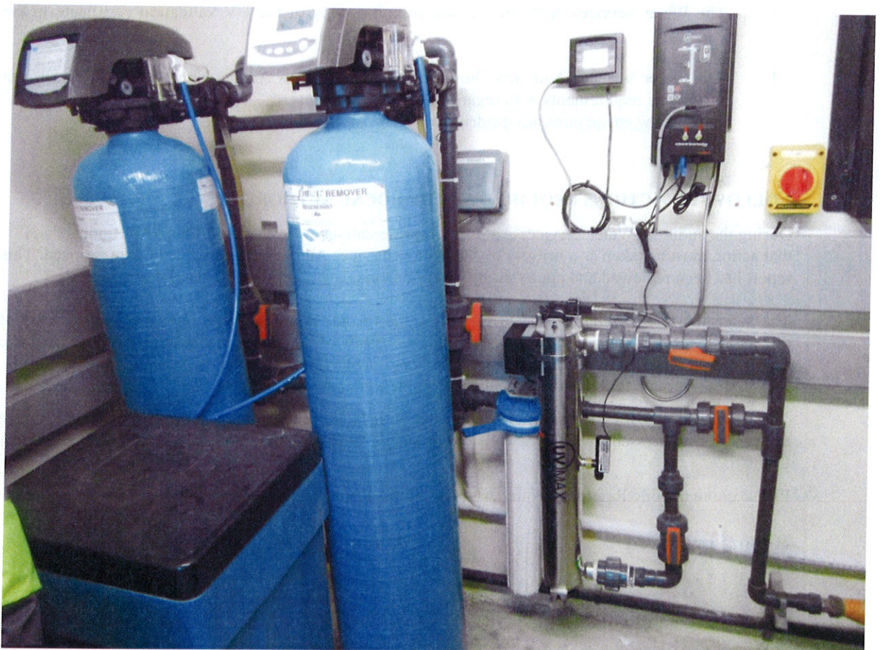
Photograph No. 2: Nitrate Removal System
