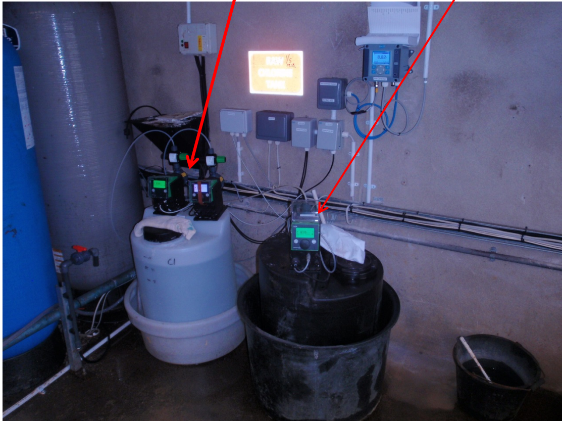
Photograph 1: Oxidation / pre chlorination dosing via duty/standby pumps. This dosing system is not connected to a chlorine residual monitor. Sodium Hydroxide (pH adjustment) is dosed via a duty pump there is no standby dosing pump. Neither system is alarmed or connected to a recording device.
