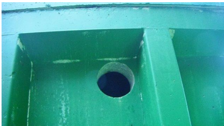
Photograph 2: Unmeshed vents allowing access to treated water reservoir.
