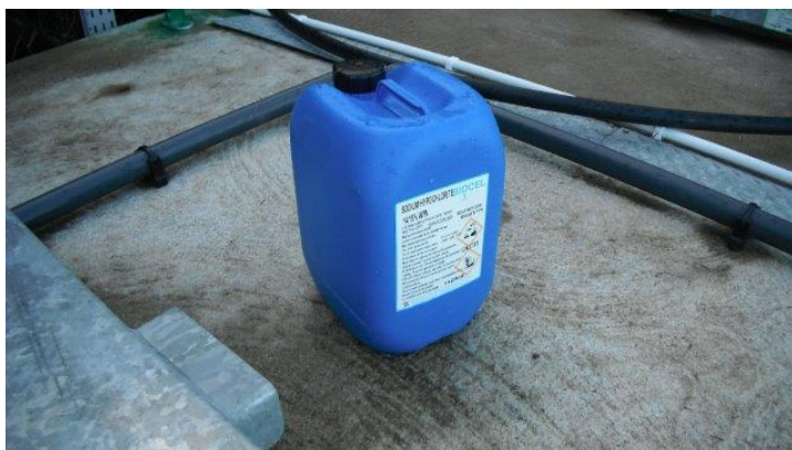
Photograph 1: Drum of sodium hypochlorite on roof of reservoir.
