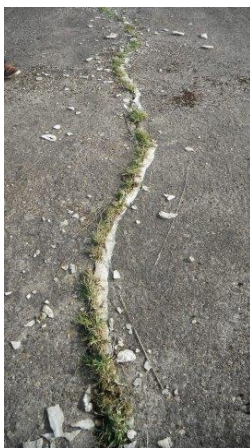
Photograph 1: Repaired crack in reservoir roof in need of further repairs.
