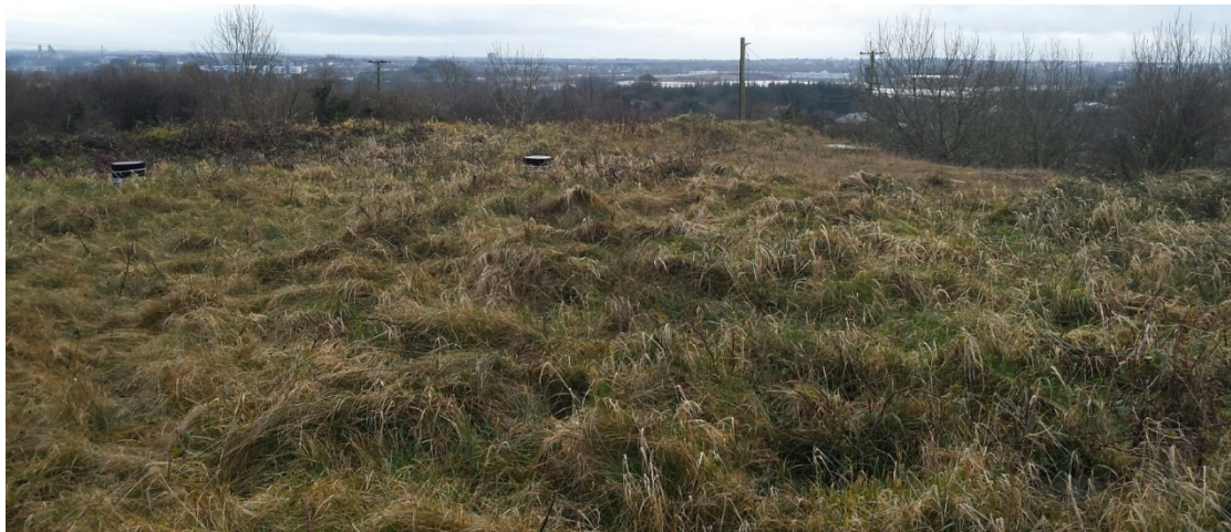
Photo 3 Overgrowth of vegetation on the roof of Coosan Reservoir
