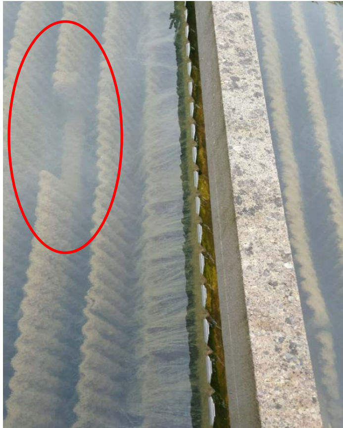
Photo 1 Sludge on clarifier and broken lamellae plate (circled)
