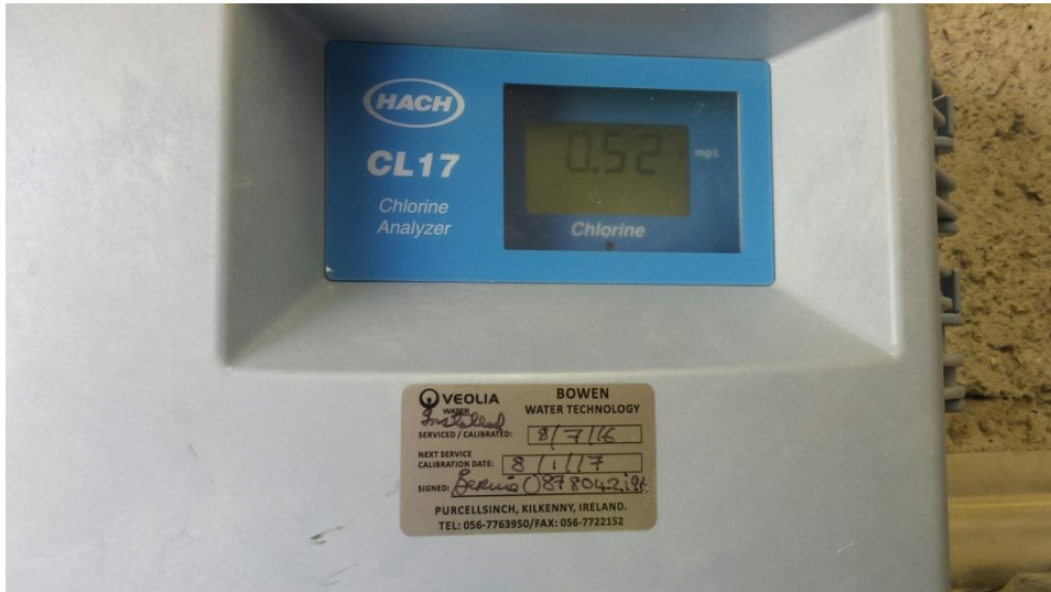
Photo 2: Label on chlorine monitor shows that calibration is overdue since 08/01/17.
