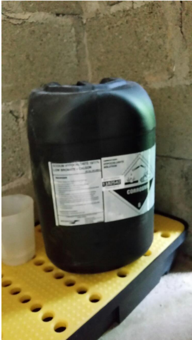
Photograph 3: Sodium Hypochlorite drum within bund
