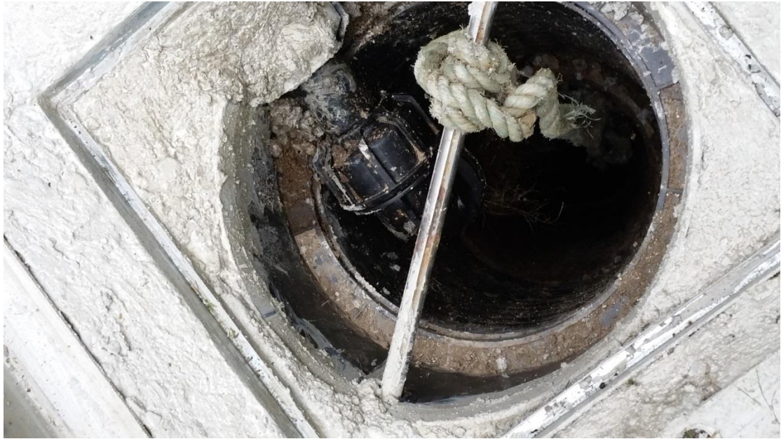
Picture No1: Main Bore Hole at Glynn Treatment plant not capped.
