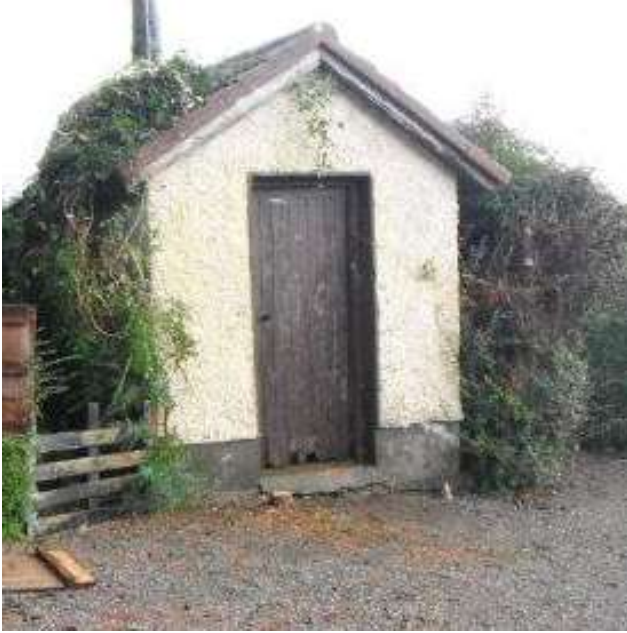
Photograph 1: Oldcourt pumphouse in need of repairs
