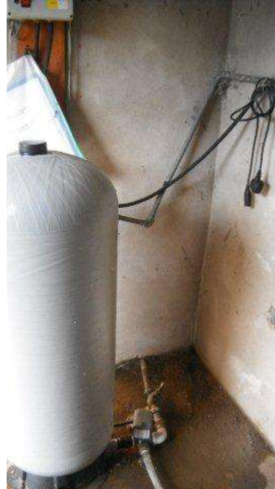
Photograph 3: Pressure vessel inside pumphouse and water from leaking roof on floor.
