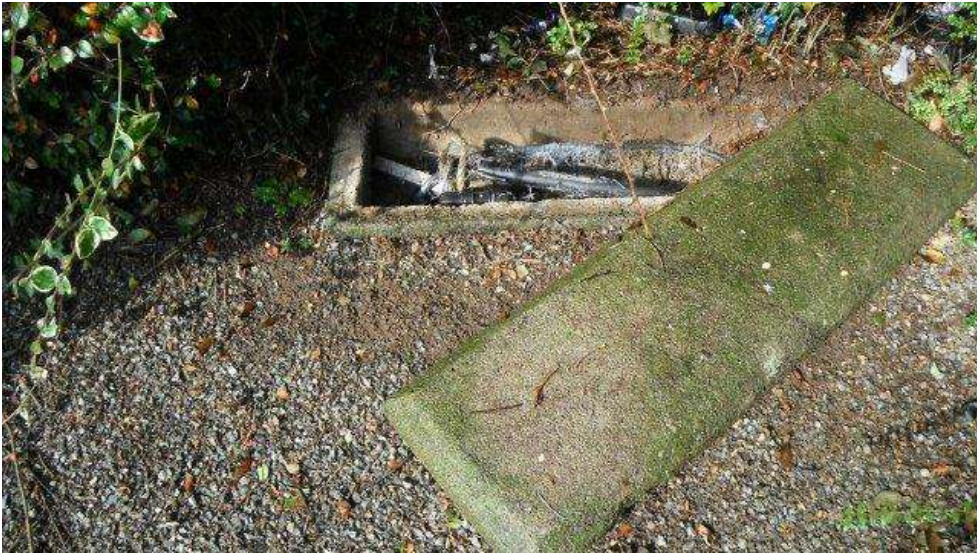
Photograph 2: Wellhead with concrete slab cover and potential entry of surface water to well
