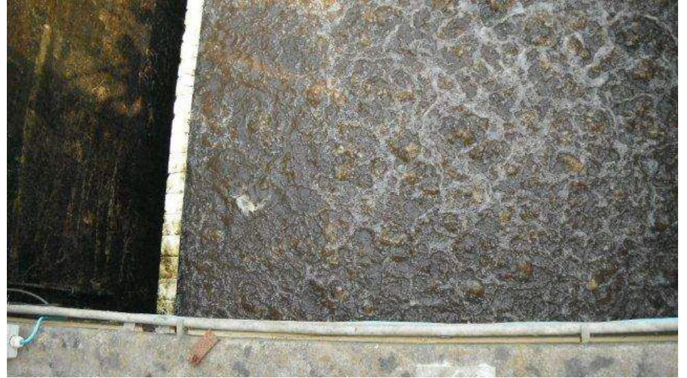
Photograph 3: Uneven air scour on Filter 1
