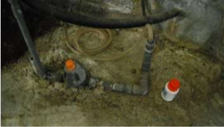
Photograph 1: Aluminium sulphate injection point – liable to being damaged by plant
