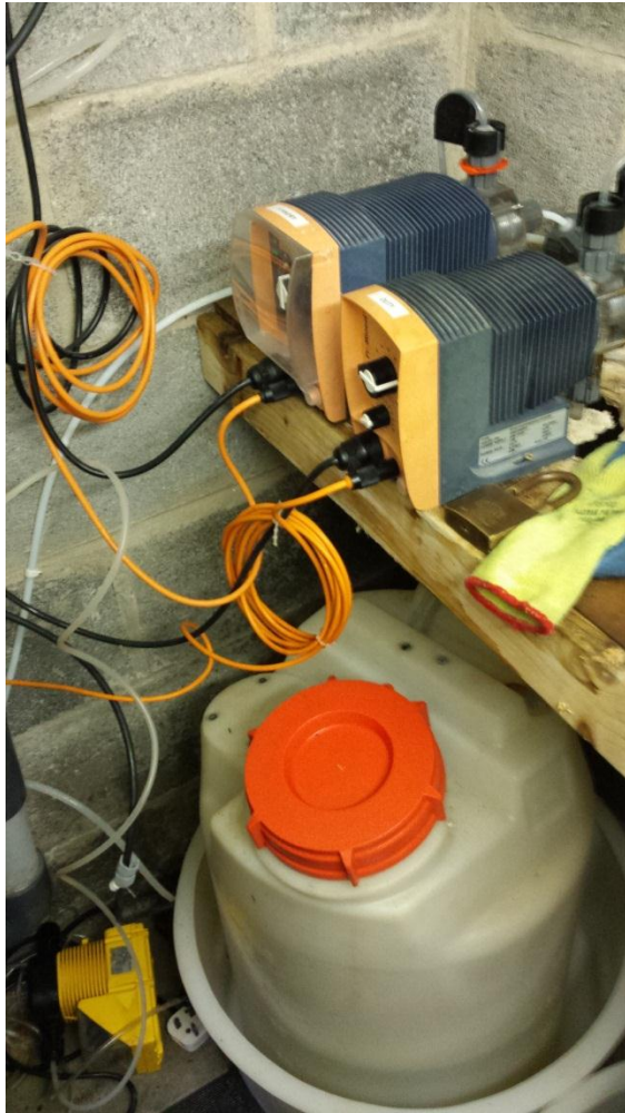
Photo 3: Duty and standby chlorine dosing pumps.
