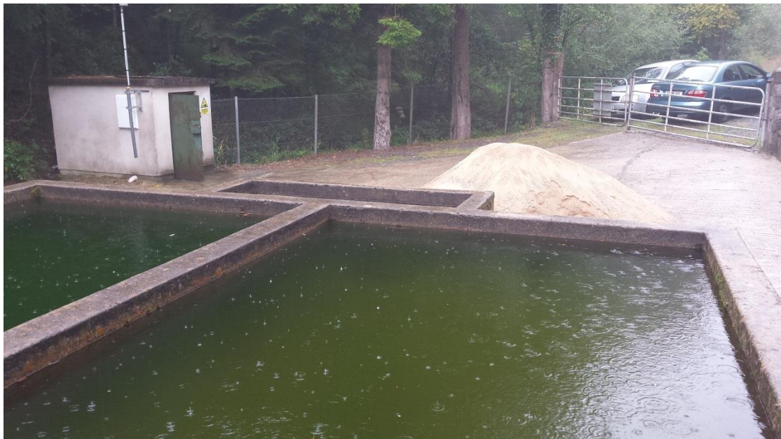
Photo 2: Two slow sand filters and plant control room.
