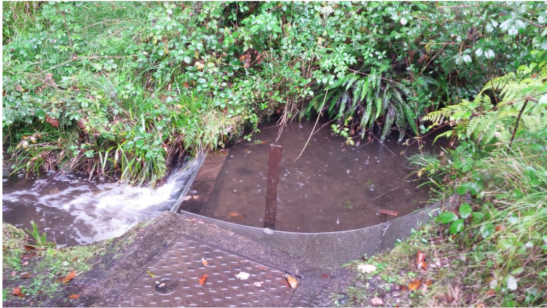
Photo 1: Stream source and intake manhole adjacent to Barnbawn water treatment plant.
