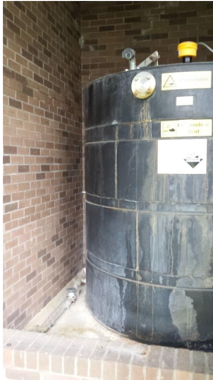
Photo 1. Fluoride Bulk Storage Tank.
