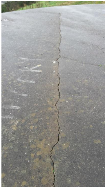
Photo 4. Crack observed in the roof of the Seacrest Reservoir.
