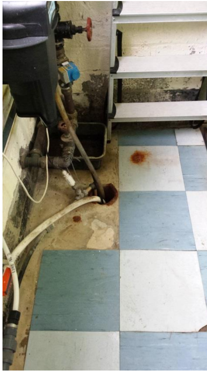
Photo 1. Hole observed in the floor of the Cronroe WTP leading to the filtered water channel.
