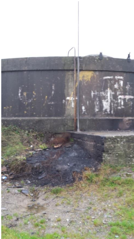
Photo 3. Evidence of burning at the Seacrest Reservoir.
