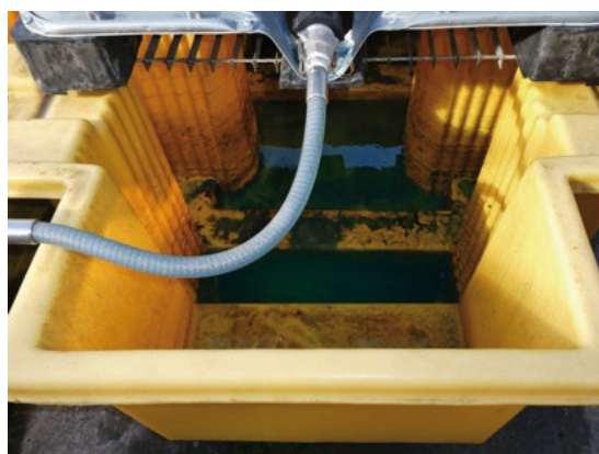
Figure 3 Outdoor bund containing liquid
