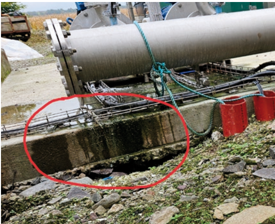
Figure 4 Leaking process pipe (leaked material indicated by red oval)
