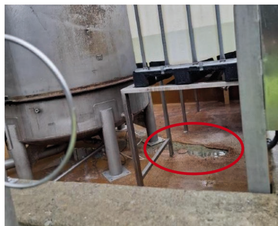
Figure 2 Bund floor in disrepair (red oval)
