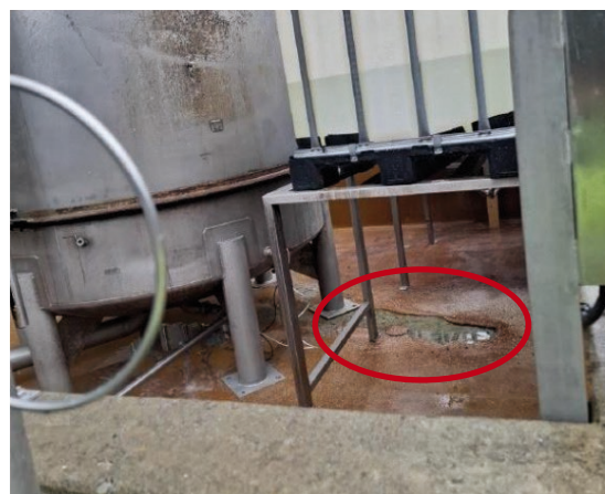
Figure 2 Bund floor in disrepair (red oval)
