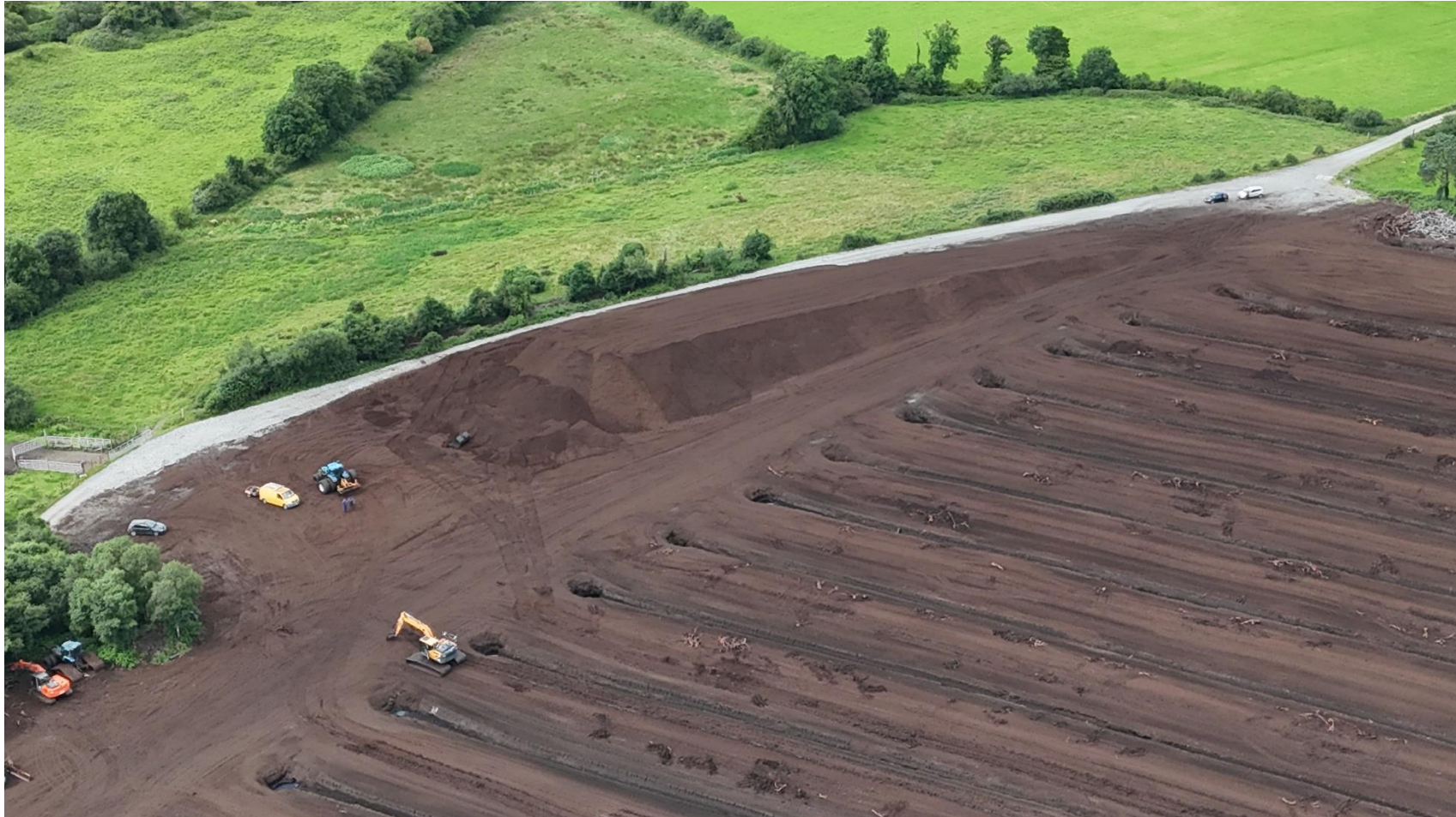
Photo 3: Significant stockpile of peat noted at the loading area.
