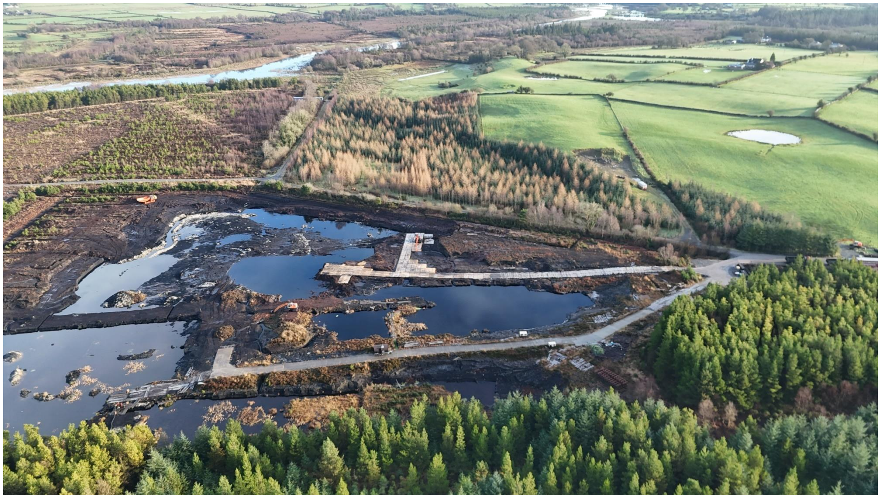
Photo 2: Photo showing road network on the peatland, note also excavators and machinery.
