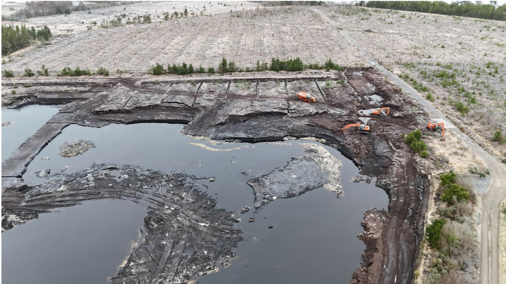
Photo 2: Three excavators and a machine for transporting peat noted at the peatland.
