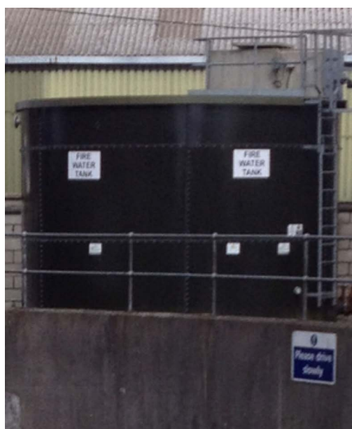
Figure 4.2 Static fire-fighting water supply tank
