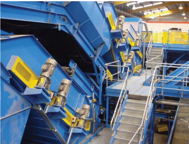
Figure 3.1 Complex WTS processing area (Photo: courtesy of Designer Group)
