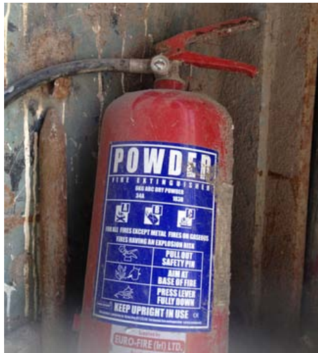
Figure 4.1 Poorly maintained fire extinguisher
