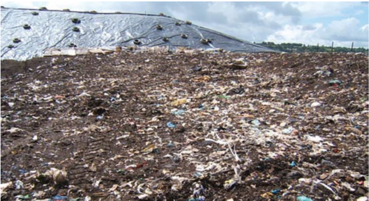
Figure 2 Eroded Cover At Landfill
