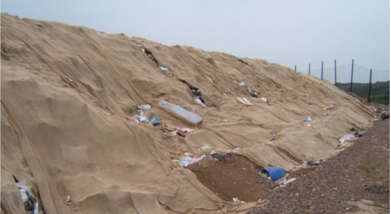
Figure 3 Inappropriate Covering Of Side Slopes
