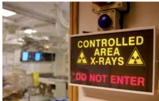
Photo 6.3(b) Radiation warning lights and signs
