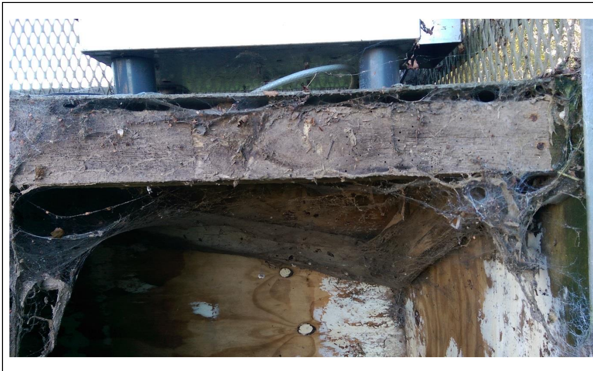
Figure 3-2 Rotting wood supporting brace
