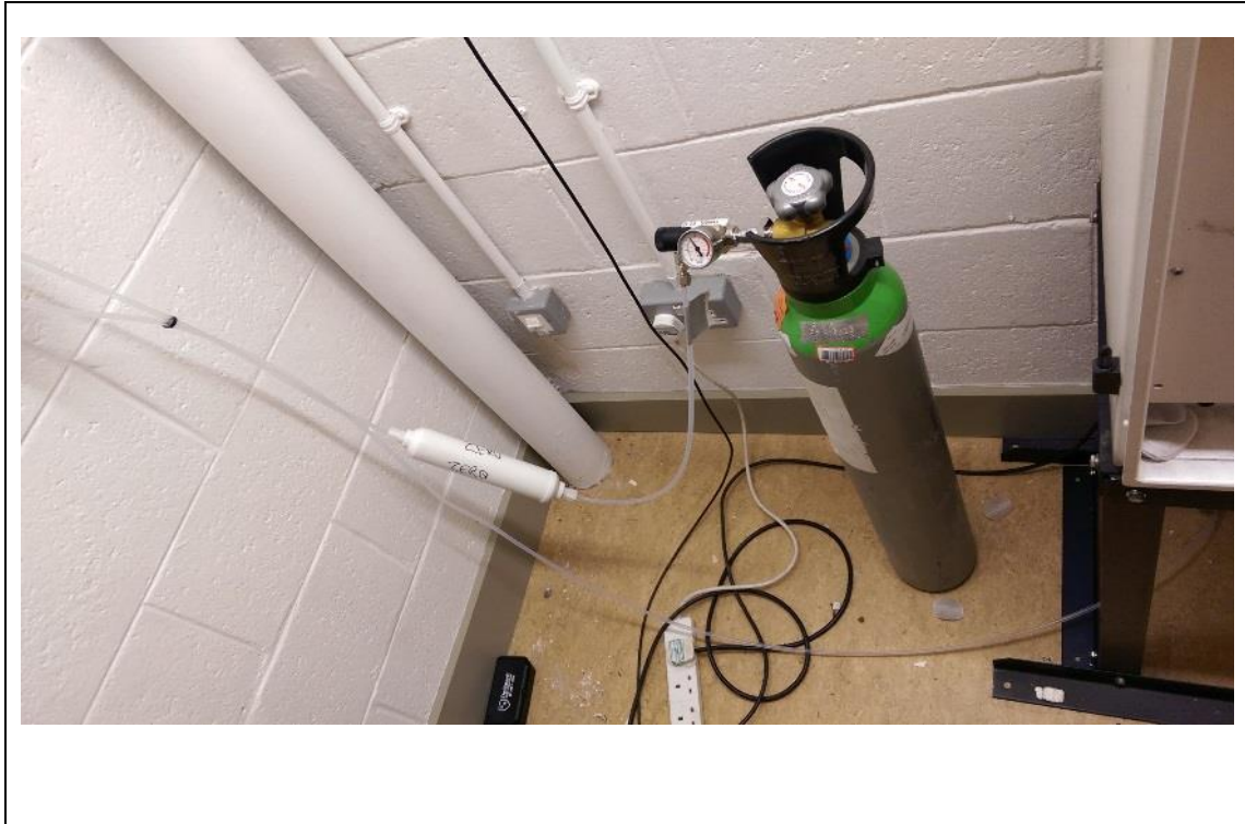
Figure 3-4 No restraint on cylinder
