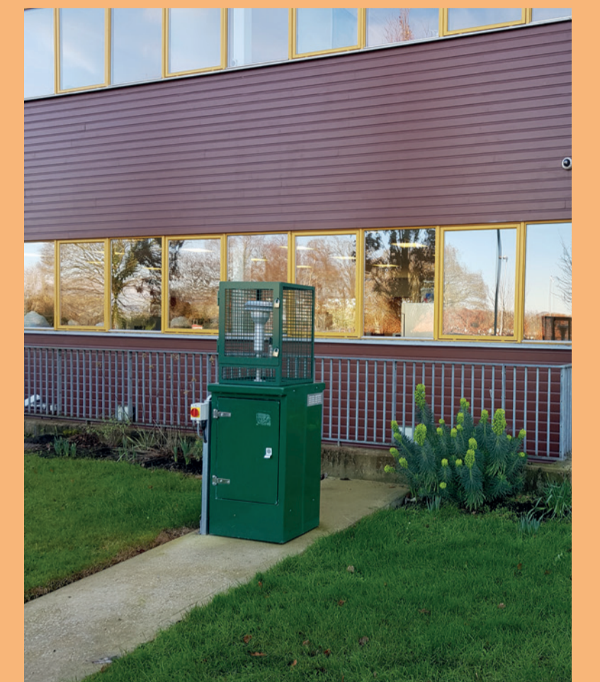
Air Quality Monitor at Seville Lodge in Kilkenny.
