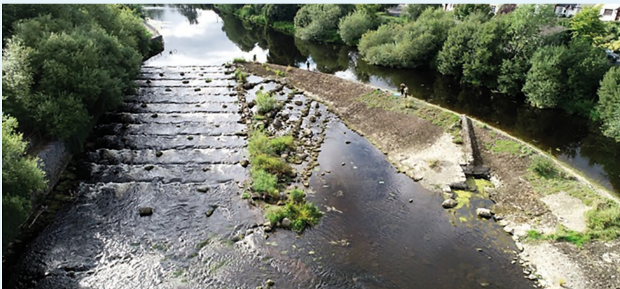
A barrier that has been ameliorated by the construction of a fish passage
