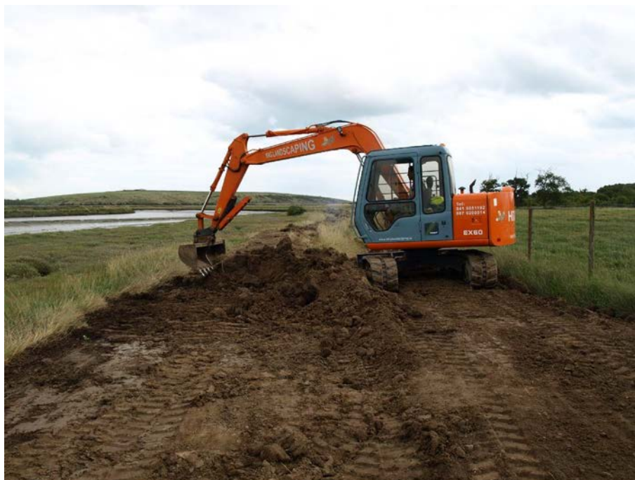
Figure 6.3. Flood embankment removal at the Rogerstown Estuary to restore the natural saltmarsh habitat and floodplain functioning. Source: Final County Council (2022a).
