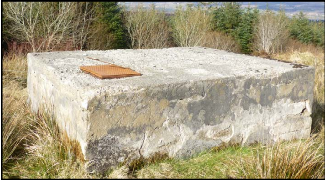
Figure G3.15. Glenfarne G.W.S. Water holding chamber only. Unable to access spring source.
