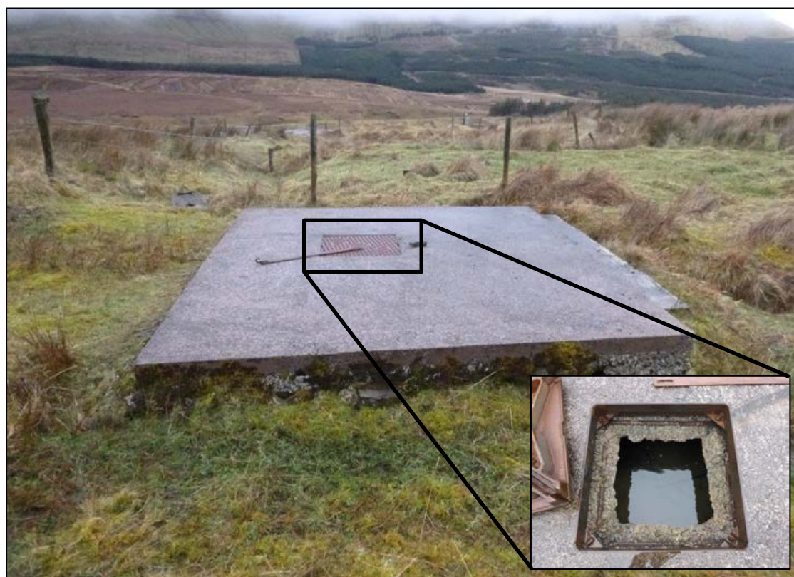
Figure G3.2. Ballintrillick G.W.S. spring collecting chamber.
