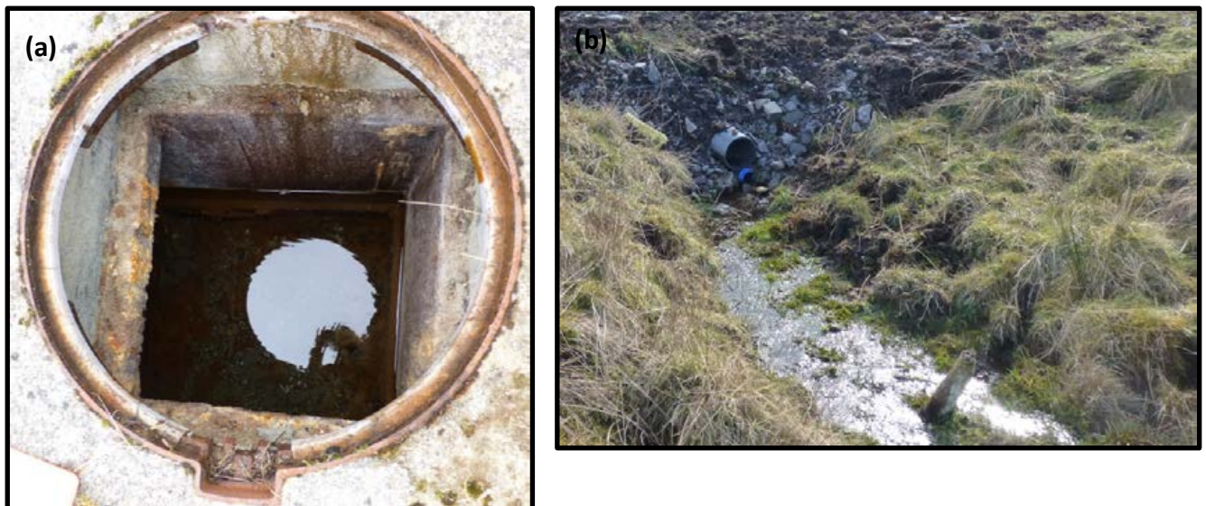
Figure G3.22. Rossinver P.W.S. showing (a) spring chamber and (b) piped overflow.
