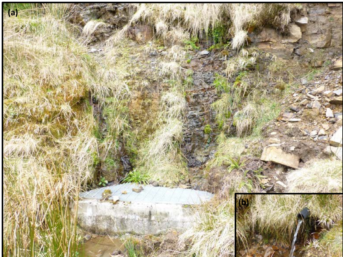
Figure G3.23. Aghacashel G.W.S. showing (a) spring water flowing down rock face to harvesting tank and (b) piped overflow.
