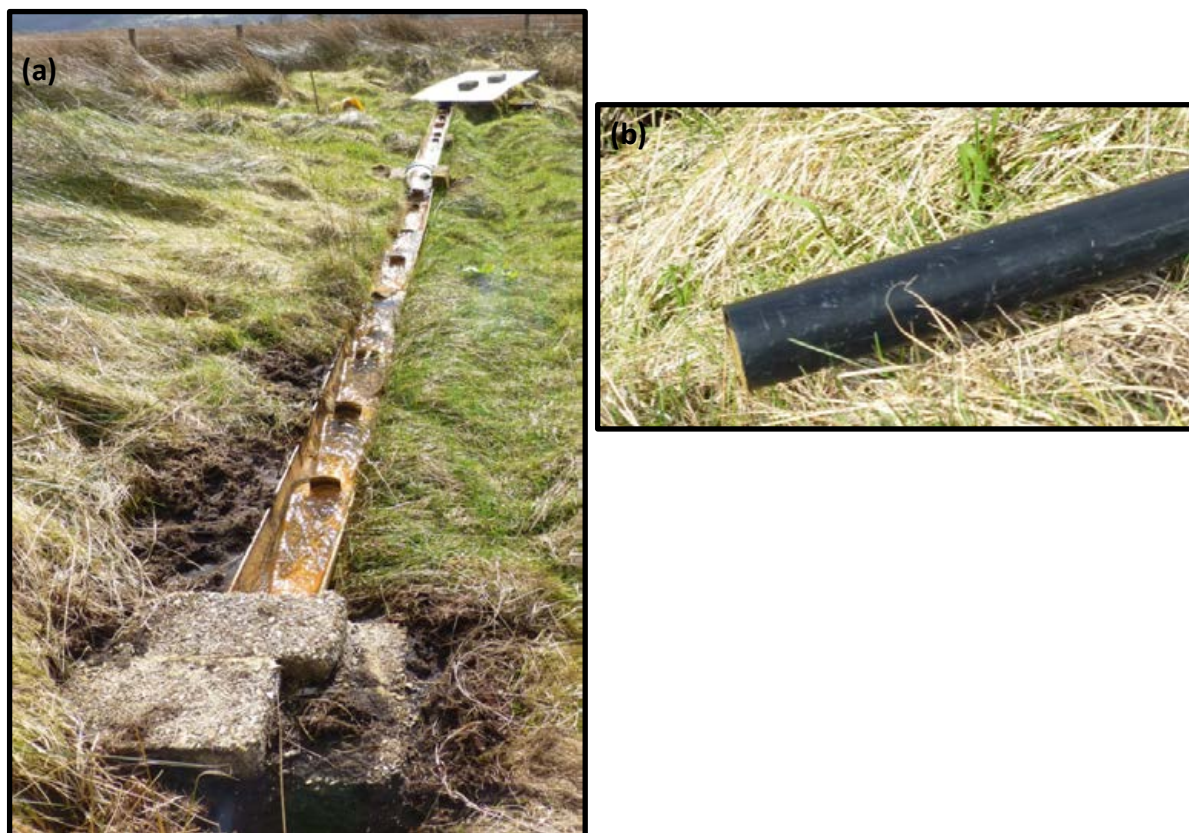
Figure G3.25. Upper Aughagrainia G.W.S. showing (a) water channelled from spring source and (b) dry overflow pipe.
