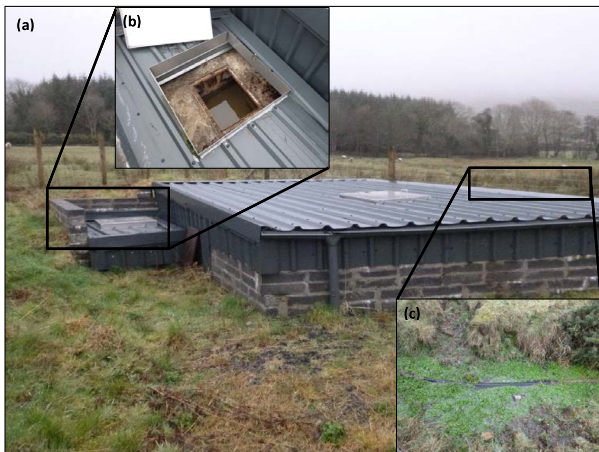
Figure G3.4. Benbulbin G.W.S. (a) spring chamber, (b) the spring source and (c) unpiped overflow.
