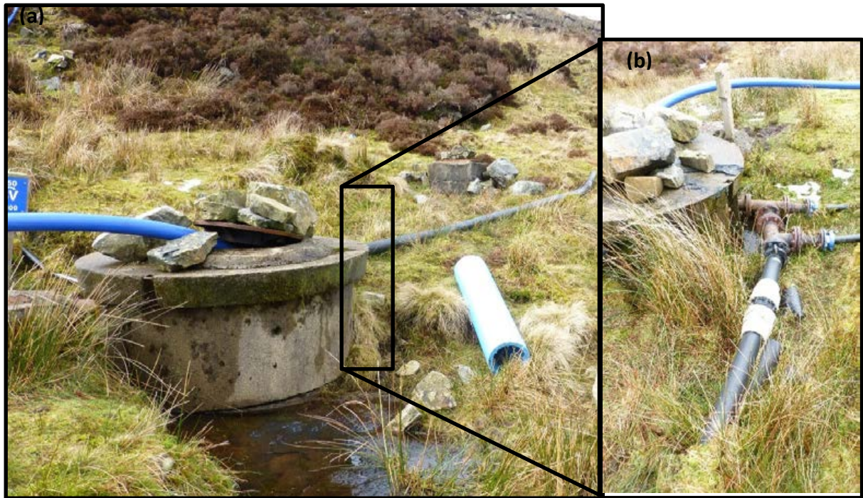
Figure G3.6. Corlough G.W.S. showing (a) view from front and (b) view from back of the spring chamber to which all springs flow before being pumped.
