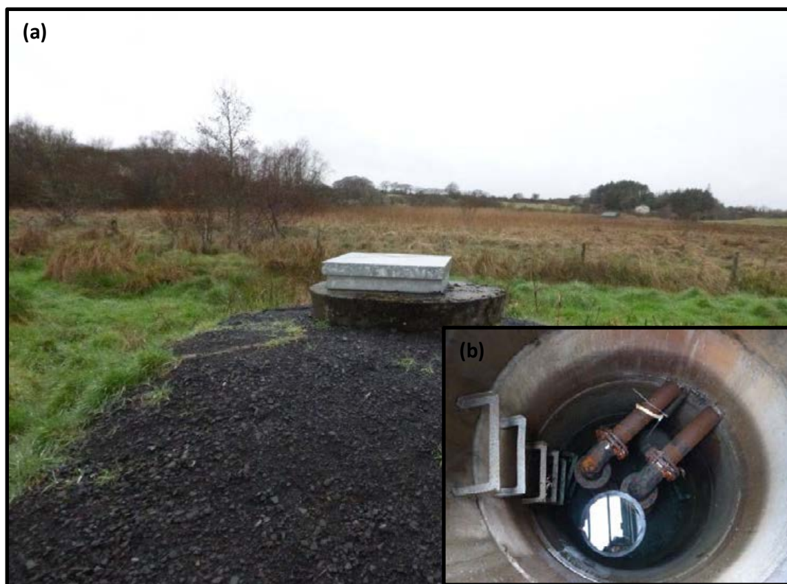
Figure G3.20. Riverstown G.W.S. showing the (a) external view, and (b) internal view, of the spring chamber.
