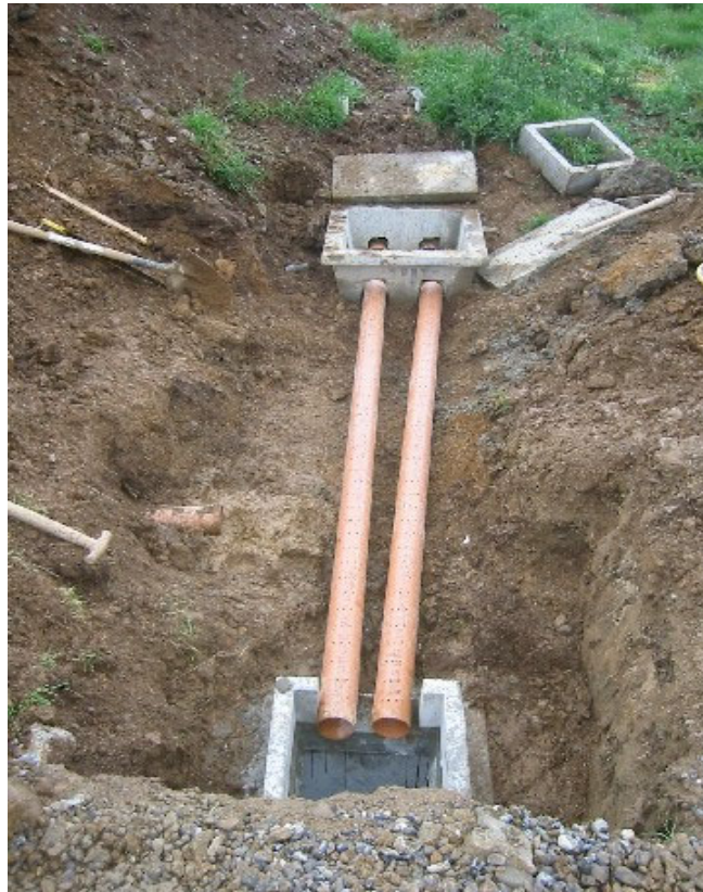
Figure 3.11 Effluent diverted into pump sump
