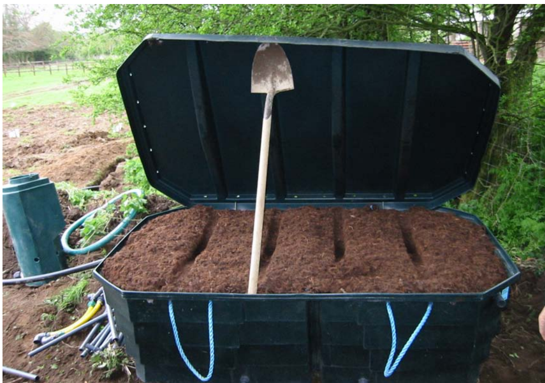
Figure 3.2 Open Puraflo ® module containing fibrous peat media. Note aeration holes along sides of lid and also the collection sump in left of photograph.
