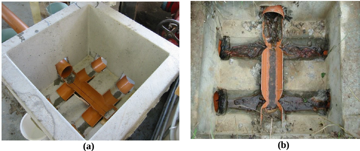
Figure 3.8 (a) Modification to standard distribution box and (b) Installed modification – note the occurrence of some deposition under field condition.
