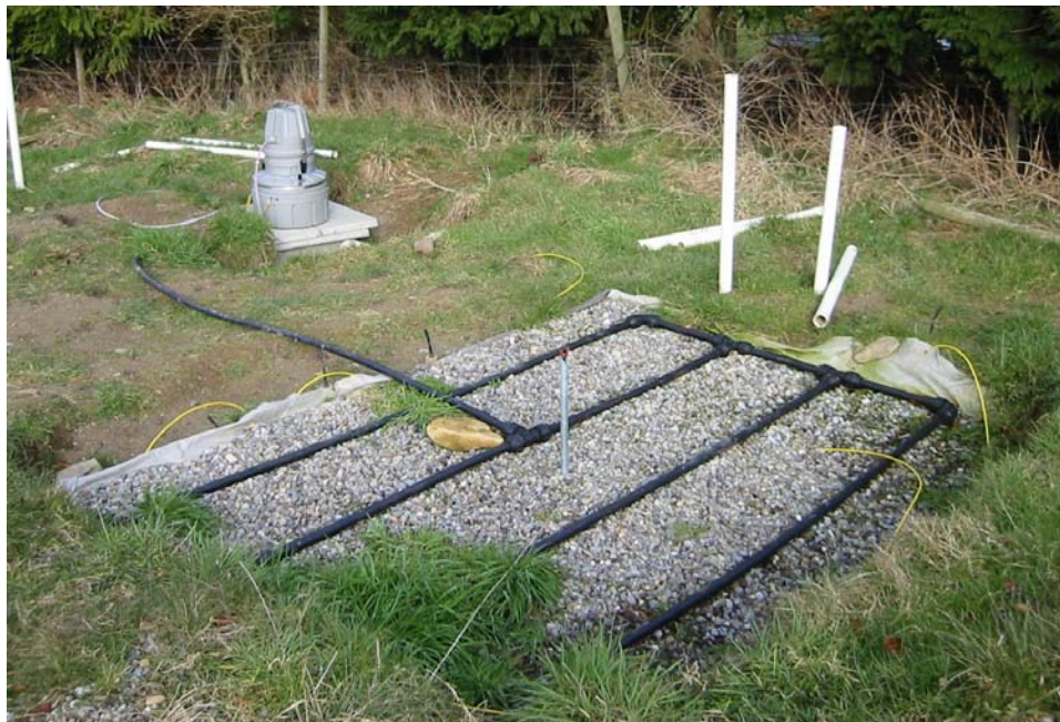
Figure 3.12 Distribution manifold placed centrally on top of sand filter
