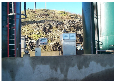
Bunded Fuel Tanks (Tarmak Ove Arkil, Rathangan, Co. Kildare)
