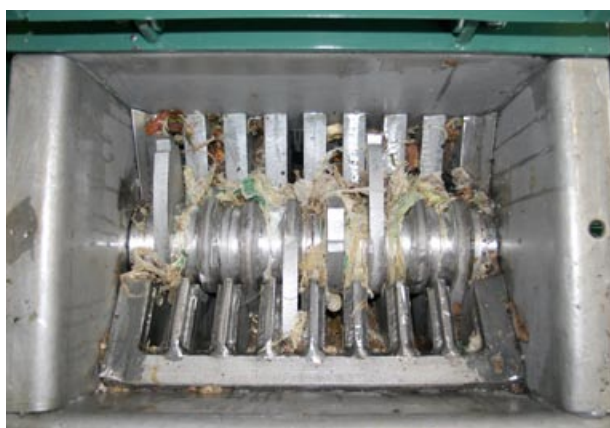
Figure 2.11: Commercial Food Waste is Macerated, Compacted and Dewatered in Onsite Unit
