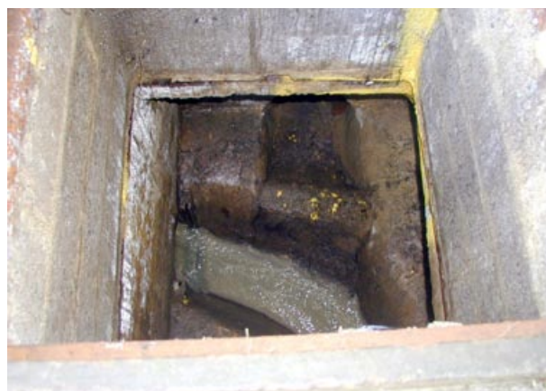
Figure 6.2: Foul Sewer and Stormwater Overflow in Irish CSO
