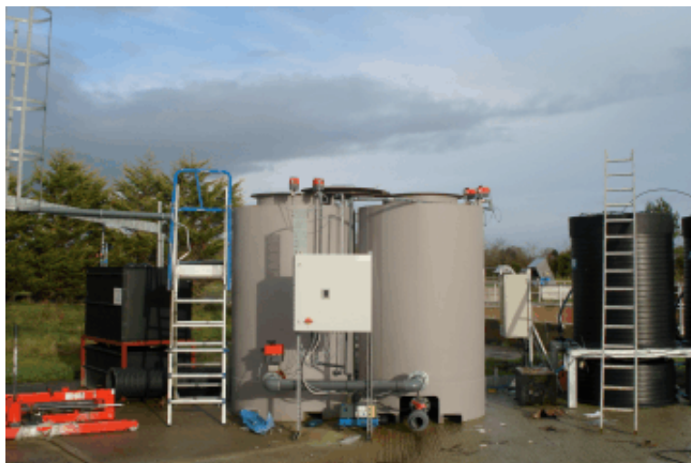
Figure 6.6. Pilot-scale air-suction flow biofilm reactor units at the Water Research Facility.
