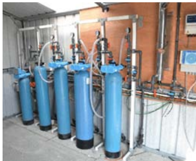
Figure 5.4. Picture of the tertiary treatment system installed at the Water Research Facility.
